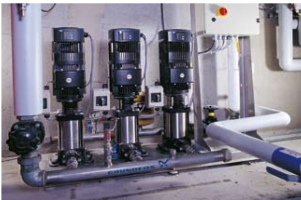
Water boosting set
